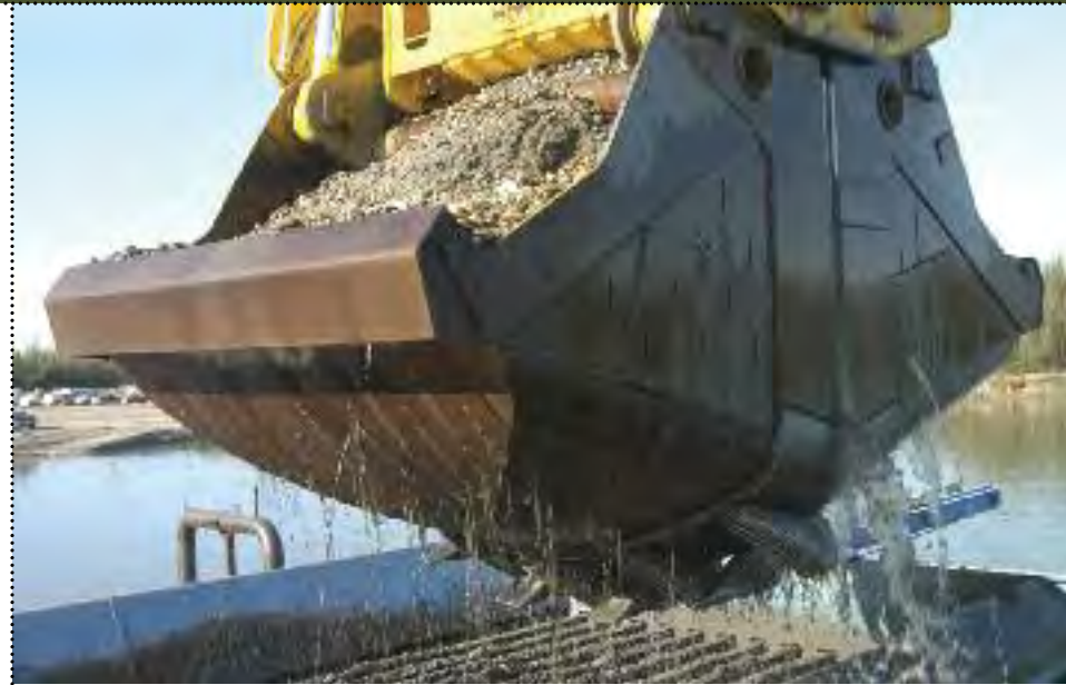
This photo shows sand and gravel extraction below the water table. Gravel is removed, leaving the water table intact.
