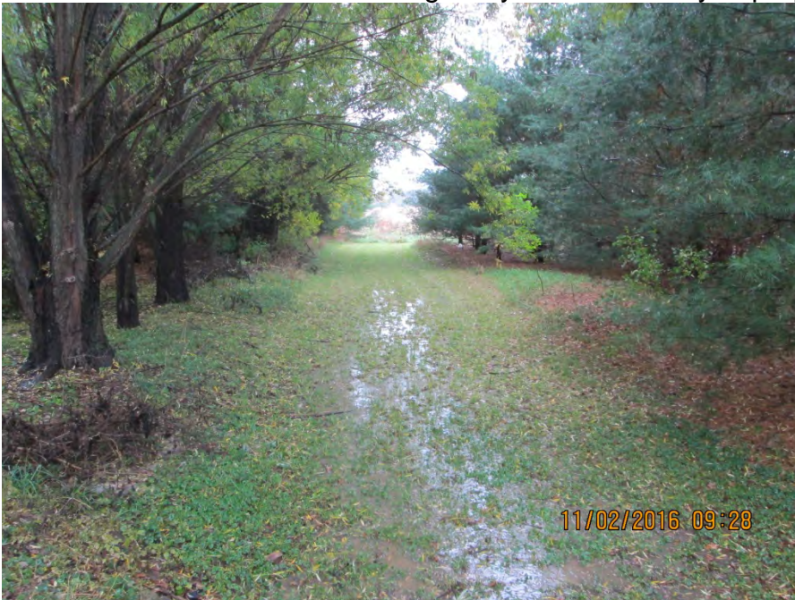
Picture shows constructed drainage way across the Payne property to the field
