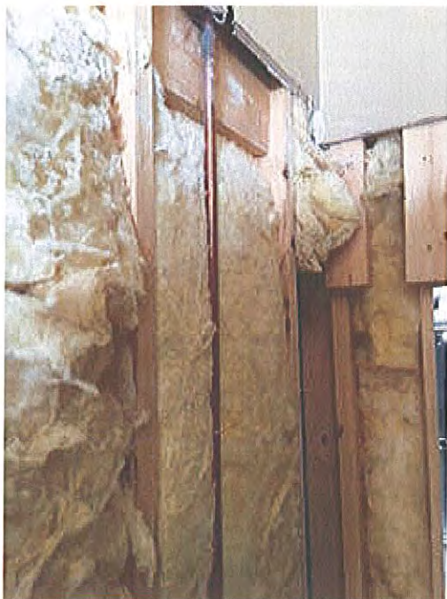
photo of removed non-operational tub
