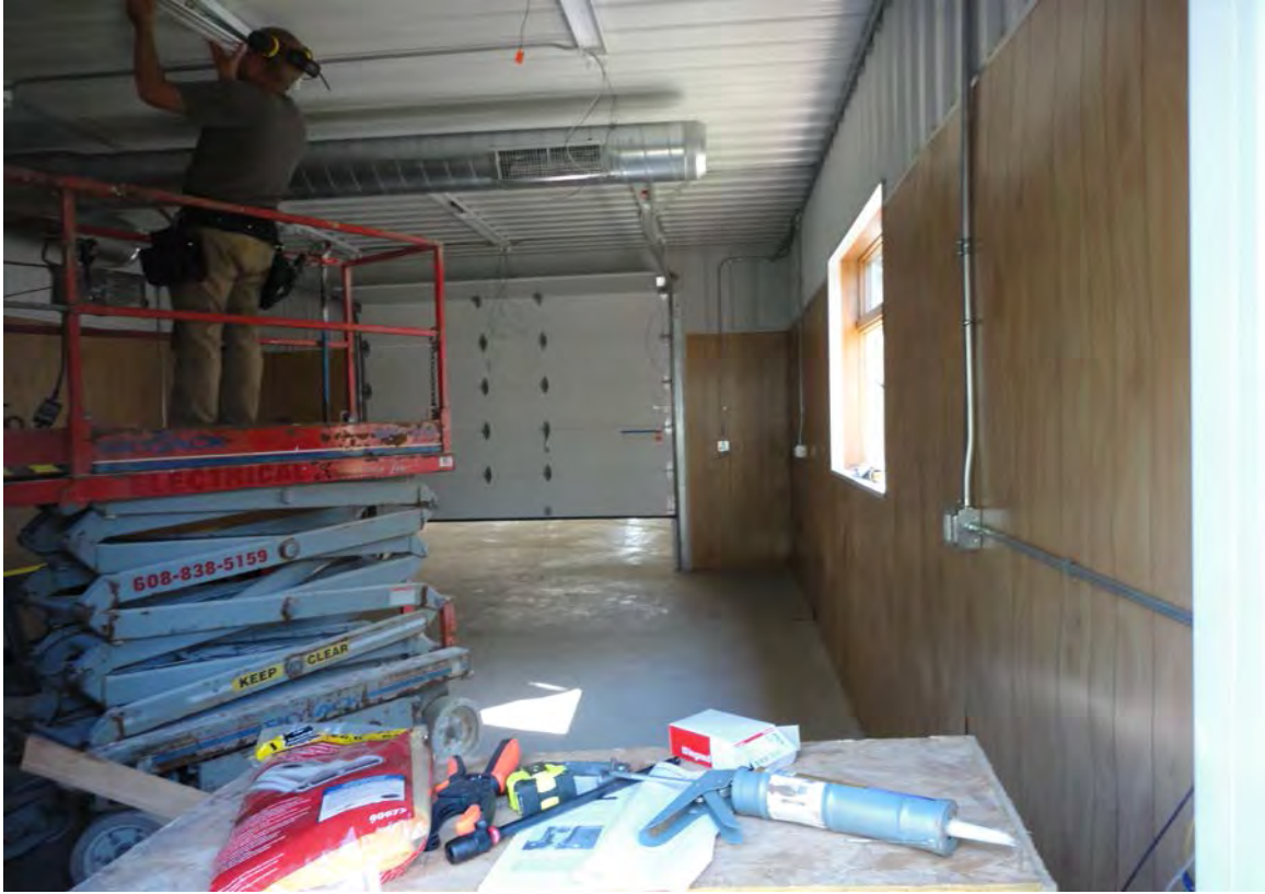
Office room – heated and electrical
