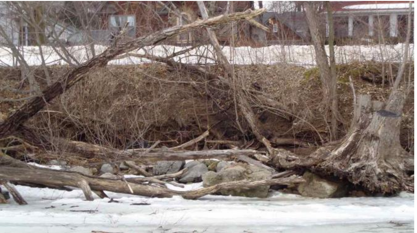
7. Example of slope collapse after trees were undercut. East of Hudson Beach.
