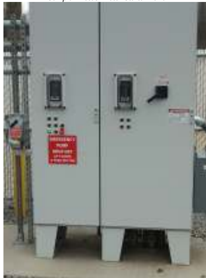
Sample Photos: Motor Starter Panel
