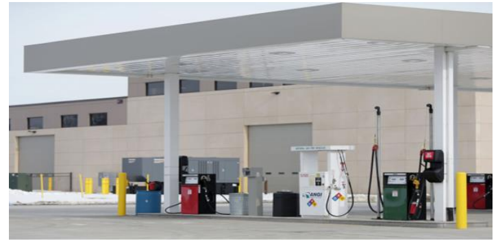
Renewable CNG Filling Station
