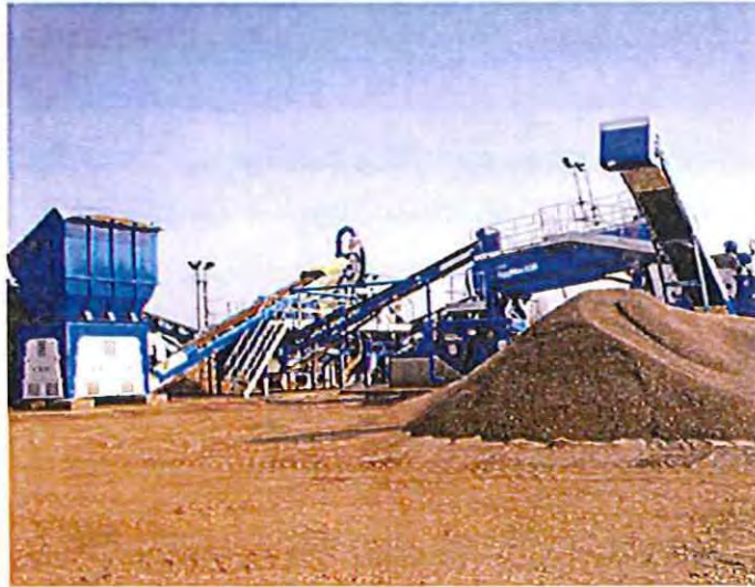
Aggregate wash plant
