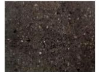
Stained concrete with fine aggregate
