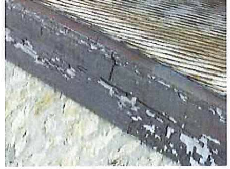
24. Rotting wood/lack of maintenance
