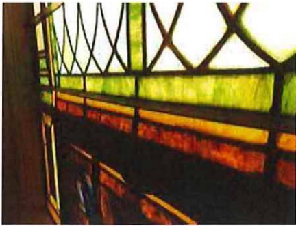
1. Loose reinforcement bar
