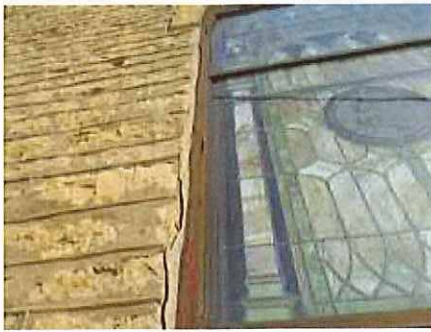
13. Lack of maintenance on tuck pointing
