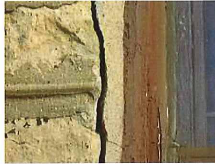
17. Lack of tuck pointing over the years from settling and expansion/contraction
