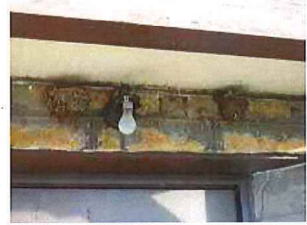
18. Lack of maintenance
