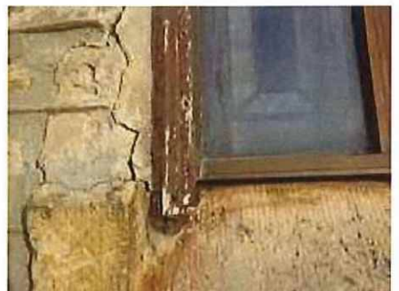
12. Rotting wood on frames due to lack of maintenance
