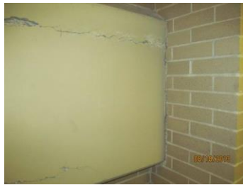
Photo 14: Stairwell structural damage
