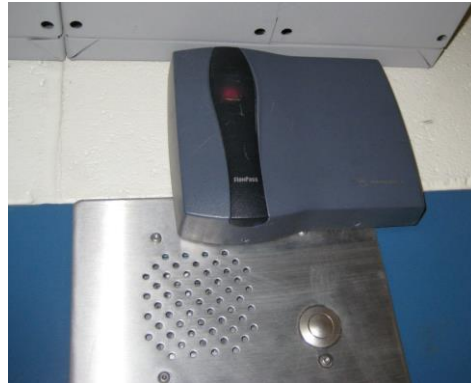
Photo 7: Proximity Card Reader
