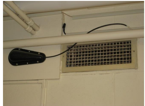
Photo 10: Internal Distribution Antenna
