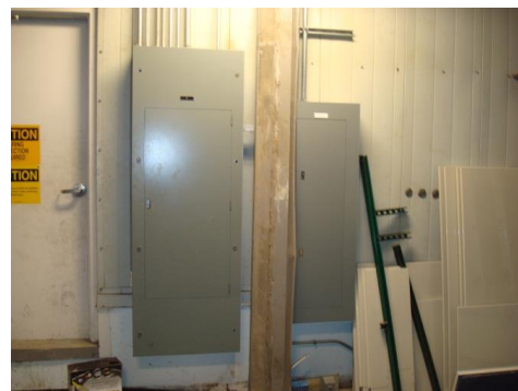
Panels WP and WPA (Penthouse Electrical Room)
