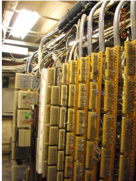
Photo 1: MDF (Main Distribution Frame)
