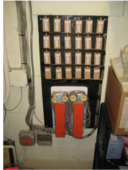
Photo 3: Inmate Telephone Cutoff Switches
