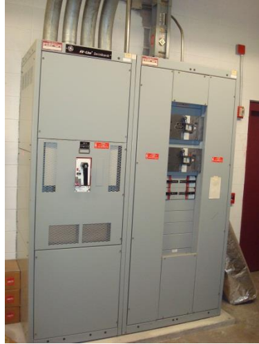
MDP-EL (Sub-Basement Electrical Room)
