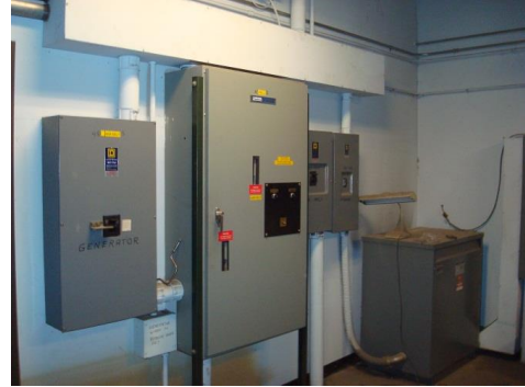
400A Enclosed Circuit Breaker and ATS #2 (East Wall Generator Room)
