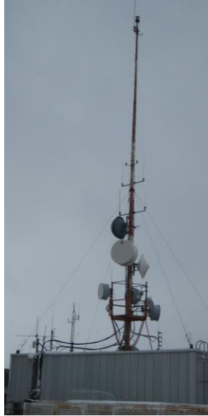
Photo 9: East Roof Antenna Array
