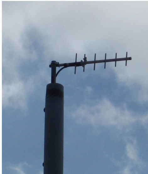
Photo 9: Exterior Yagi Antenna
