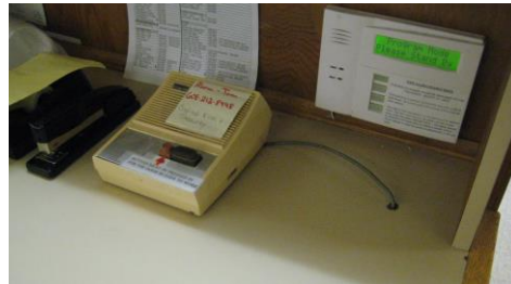
Photo 31: First Floor Watch Desk Exit Alarm and Intercom with Door Release
