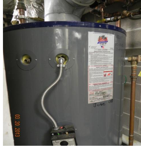
Second Floor Domestic Water Heater
