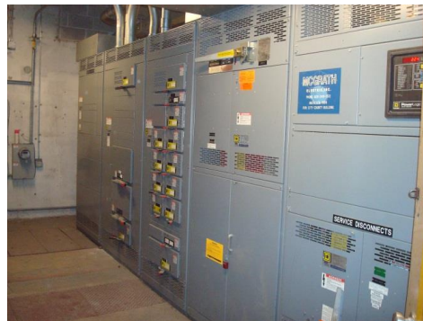
3000A, 208Y/120V West Switchboard (Ground Floor Electrical Room)
