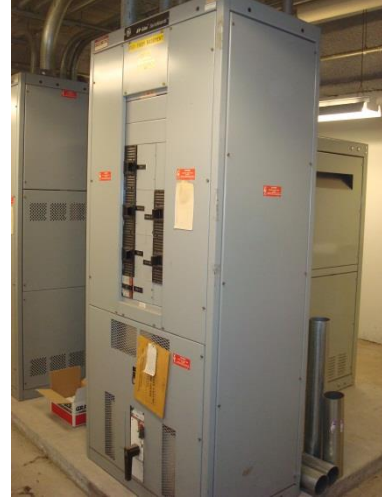
MDP-EL2 (Penthouse Electrical Room)
