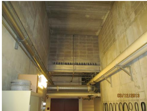
Figure 8 – Top of elevator shafts, east elevator bank on left, west elevator bank on right
