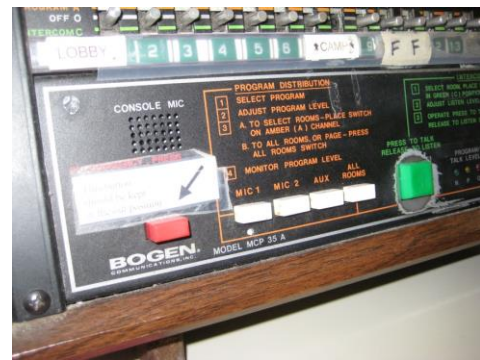
Photo 83: Second Floor Intercom System
