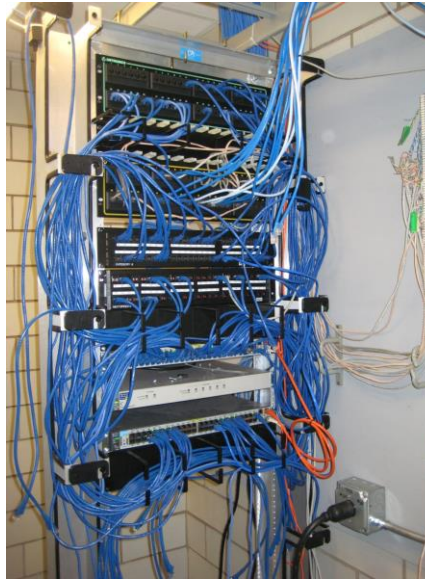
Photo 2: Seventh Floor Telecommunications Room
