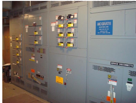
4000A, 480Y/277V Switchboard (Ground Floor Electrical Room)
