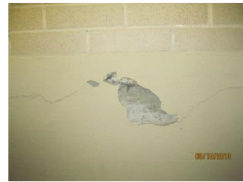
Photo 15: Stairwell structural damage
