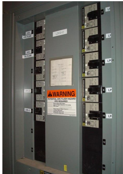
Panel LDCG-2 (Garage Level West Electrical Room)
