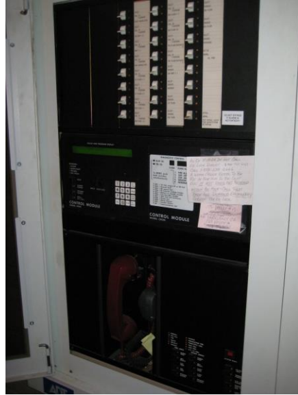
Photo 16: FACP in Central Control
