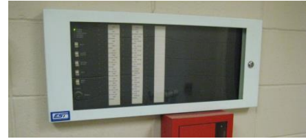
Photo 17: FAAP in Vestibule
