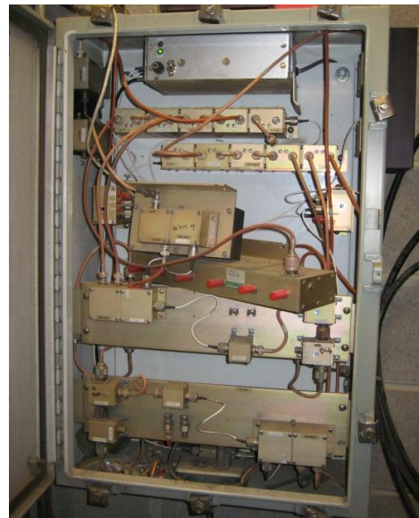
Photo 19: RF Distribution Equipment
