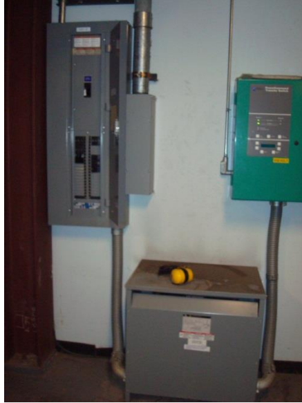
ATS #2E, 75 kVA Transformer, and Panel MDP XE (North Wall Generator Room)
