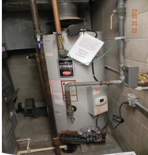
First Floor Domestic Water Heater
