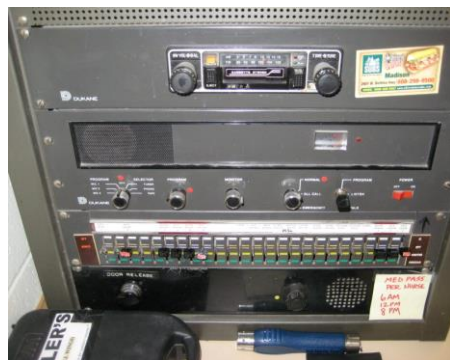
Photo 72: First Floor Intercom System
