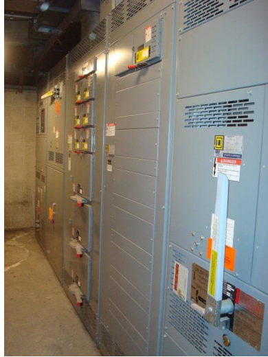
3000A, 208Y/120V East Switchboard (Ground Floor Electrical Room)
