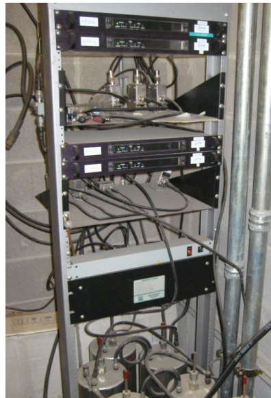
Photo 18: RF Distribution Equipment
