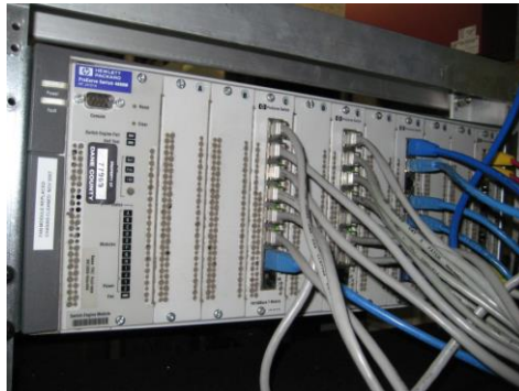
Photo 26: Second Floor Network Switch
