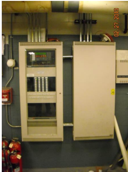
Photo 8: Building FACP (Ground Floor)
