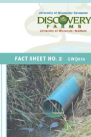
Figure 1: Tile outlet with a rodent guard.
