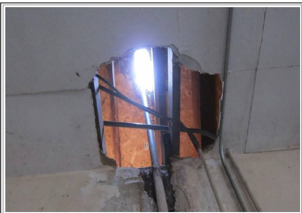
Hole in roof looking from garage
