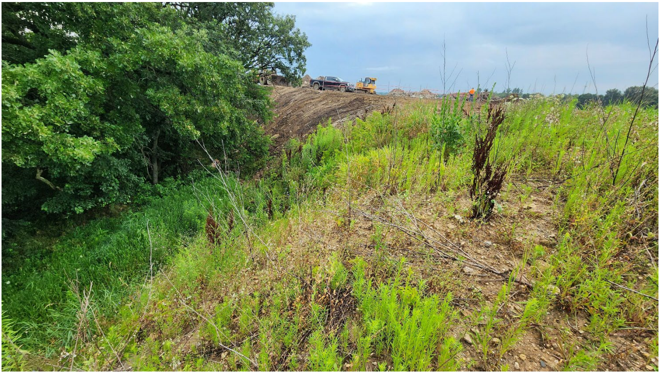
Slopes not stabilized and greater than 3:1
