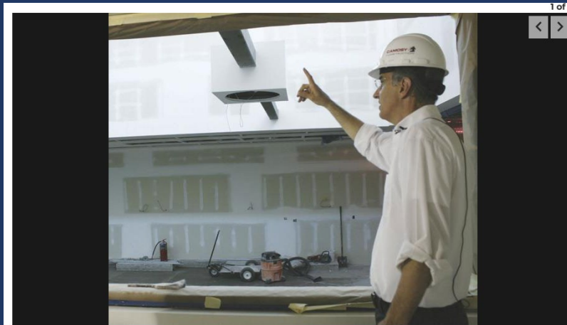
Dane County Executive Joe Parisi recently showed off the new East District Campus Project, which includes the new Medical Examiner's complex off Hwy. 12-18 Buy Now Jennifer Fetterly photo
